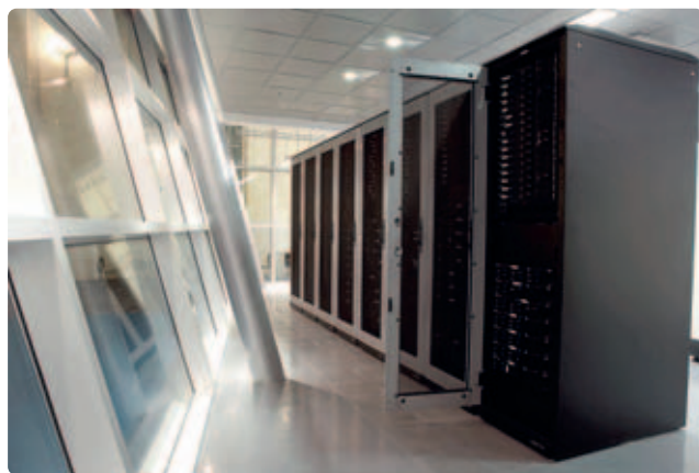
Quelle: Eaton Power Quality
